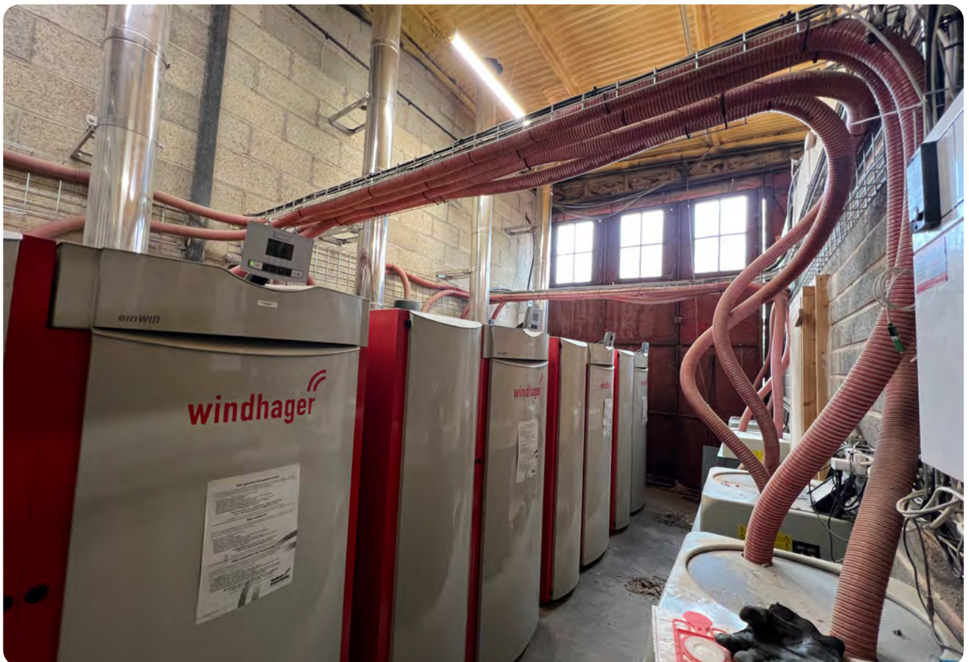
A local biomass boiler using locally sourced fuel, Cowlall.
