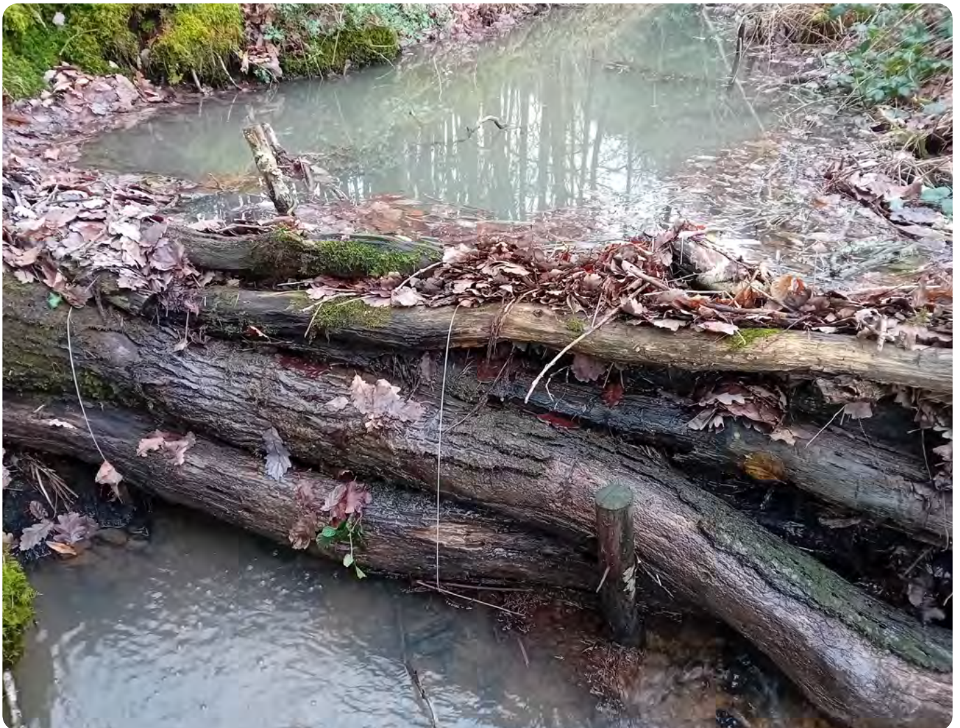
Leaky dam, Worcestershire.
