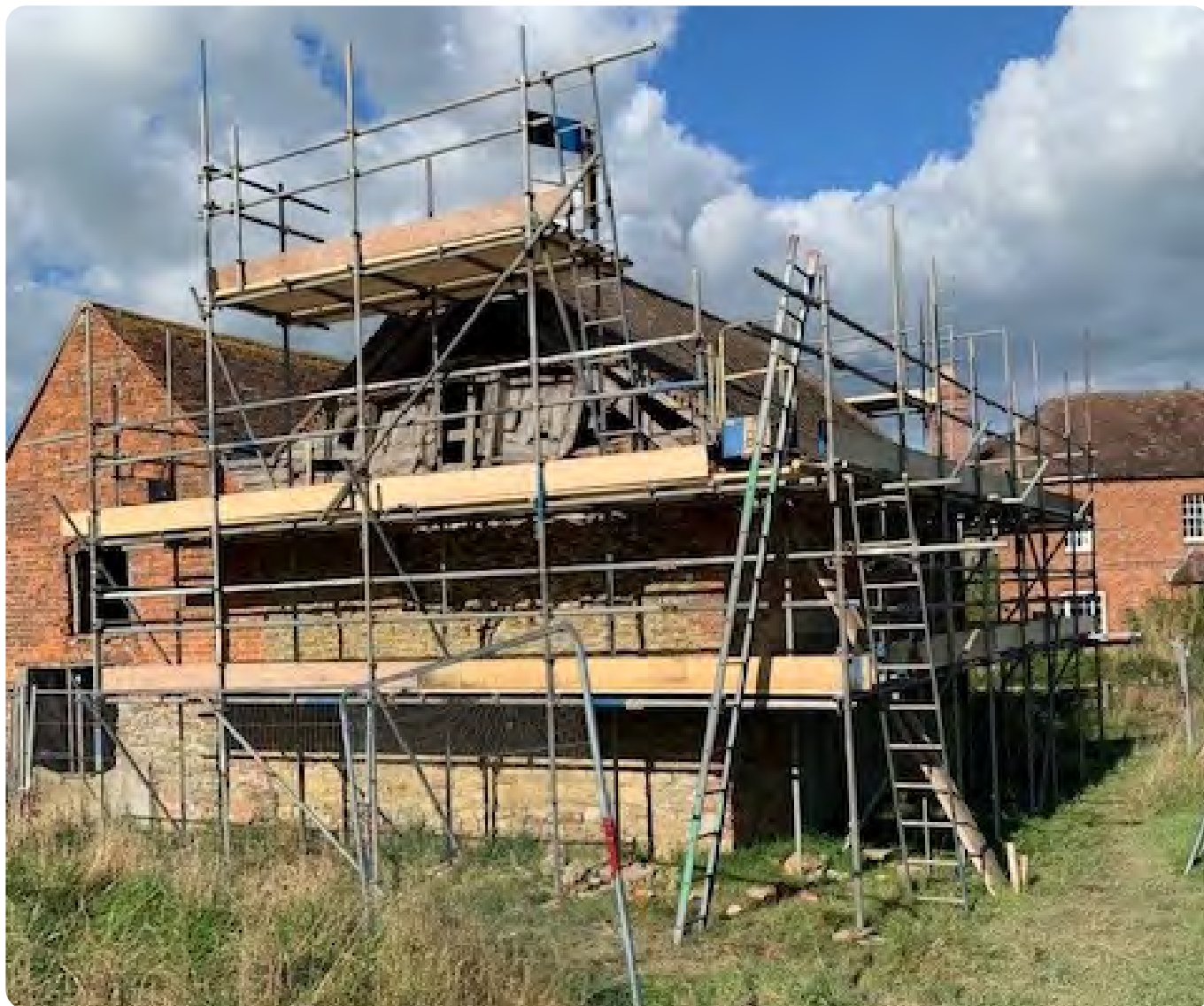
The Granary build being restored under an Historic Building Restoration Grant, Eastnor.
